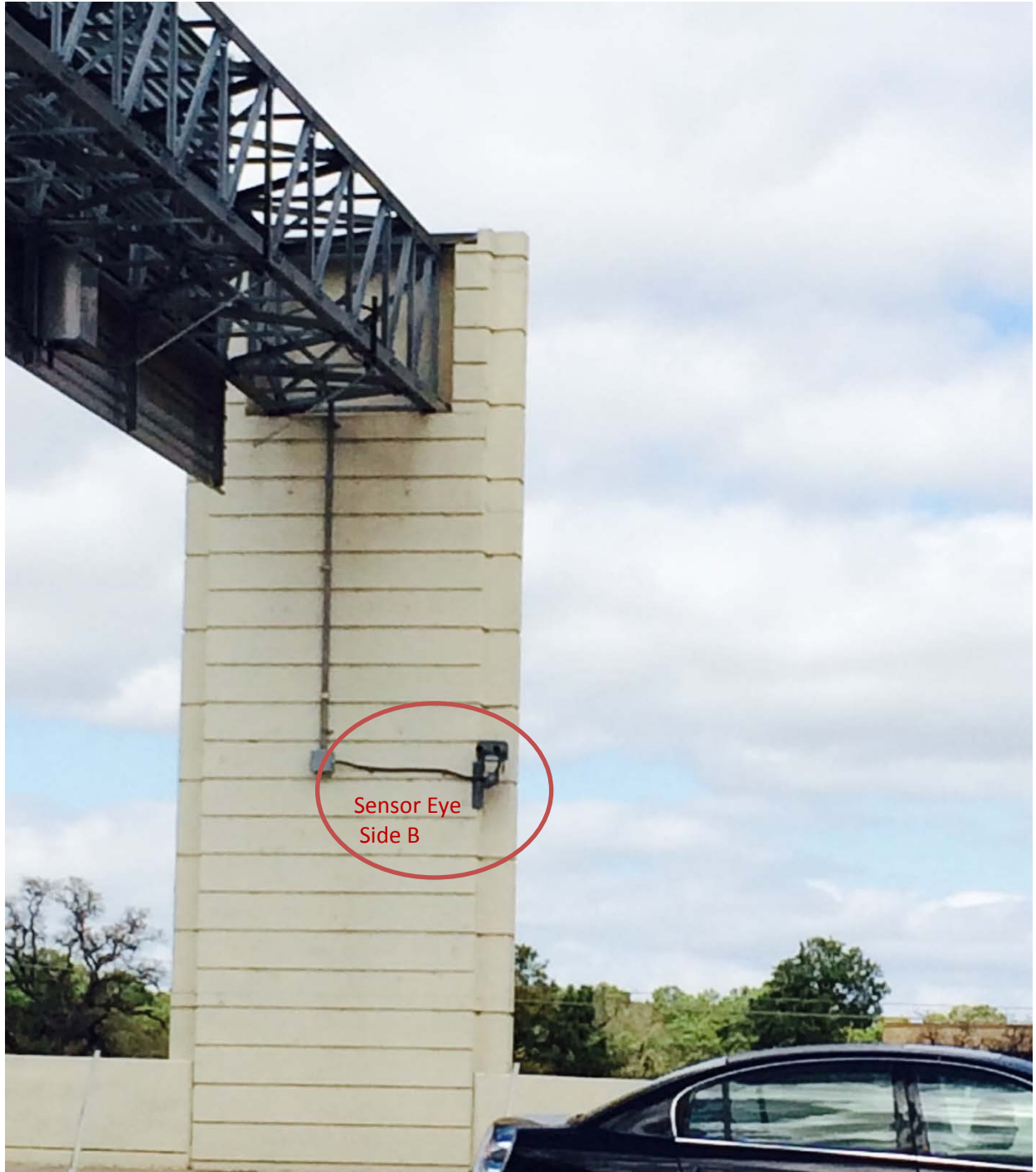
Figure 2. OVDS Components at Wirt Site (on centerline of I-10).
